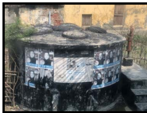
Dysfunctional pond and sand filter
